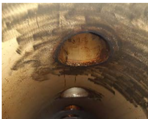
Brewery's water pipe after one year operation
